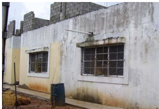
Damage caused by Tropical Storm Noel, Oct 07 07
